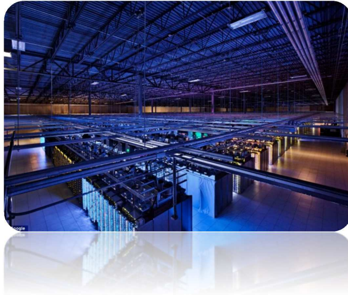
One of Google's server farms in Council Bluffs, Iowa, which provides over 115,000 square feet of space for servers running services like Search and YouTube
